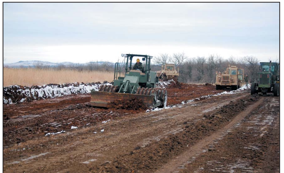
The 242nd Engineering Company, based in Coffeyville and Winfield, Kan., recently sent seven Soldiers to Crisis City at the Great Plains Joint Regional Training Center to complete a construction project. The Soldiers are building a rail bed that measures 400 feet long by 32 feet wide. Tracks will be laid on the rail bed and a train engine and several cars will be placed at the site to simulate a derailment. This completed project will give vital training on hazardous material spills and other disasters to civilian and military first responders. (Photo by Tech. Sgt. Jami Perusich)
