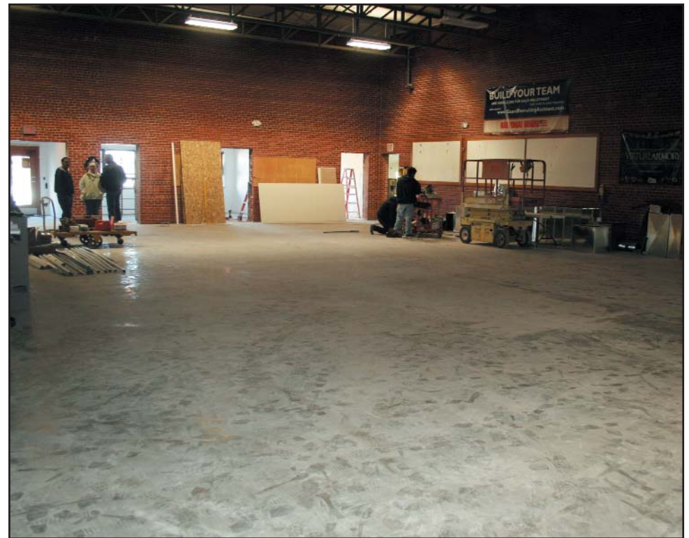
In January 2008, Maj. Gen. Tod Bunting, the adjutant general, paid a visit to the Pratt armory to check on the progress of renovations. The Kansas National Guard has 56 armories across the state. Many were constructed in the 1950s and 1960s and are in need of repair and updating. (Photo by Sharon Watson)
